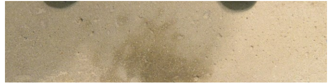
Figure 24 Concrete surfaces with shaded area and water mark (case T4-1)
