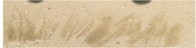
Figure 19 Concrete surfaces with water mark
