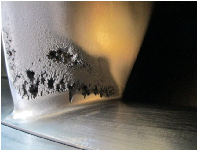
Figure 1. Cavitation blade damage on a hydroturbine runner (courtesy of the U.S. Bureau of Reclamation)
