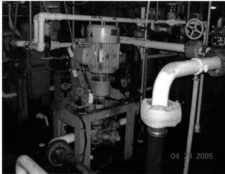
Figure 3-37: One of the fuel-oil pumps installed at the LBES.
