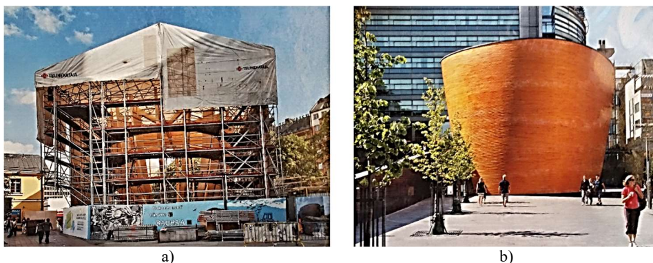
Fig. 4. a) Construction of the wooden Chapel of Silence in Kampi; b) «Kampinkappeli» Helsinki, Finland, photo by O.A. Pastukh, 2017.
