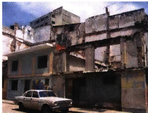
Images 4.12 + 4.13 Deteriation due to lack of maintenace
