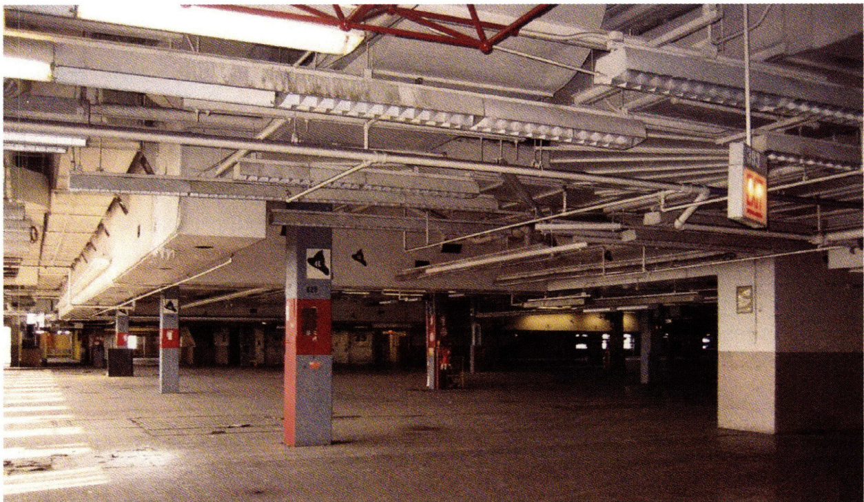
fig.35 Interior view of workspaces. Note the density of spyways, ductwork, and lighting, above.
