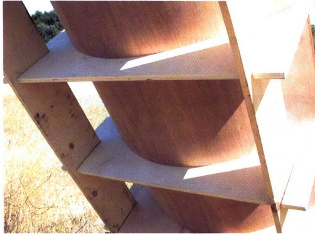
Figure 10: Stiffening the reflective surface of the trough using thin plywood screwed into the shaping ribs. (Seven Troughs, Nevada)
