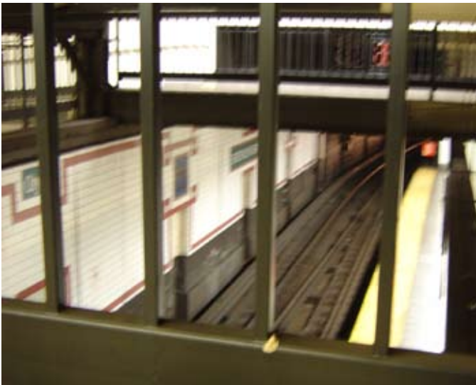
View from mezzanine to abandoned platform (after sealing off with wall in foreground)
