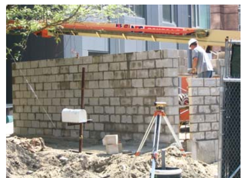
Figure 3.3 Traditional masonry construction Traditional methods of constructing masonry walls that demonstrates the limited use of curved forms
