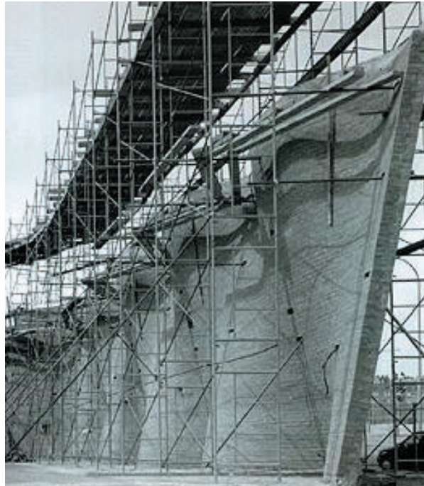
Eladio Dieste's church in Atlantido during construction. Dieste used simple construction principles to achieve his complex curved structural reinforced brick shells and walls. The image shows the physical use of lines of ruling for the construction of a brick wall. This example is an interesting variation on the paper based surfaces of Gehry. Brick allows for non developable ruled surfaces to be built both share straight lines of ruling. Dieste literally built the control polygon of the surface physically. Image: Eladio Dieste
