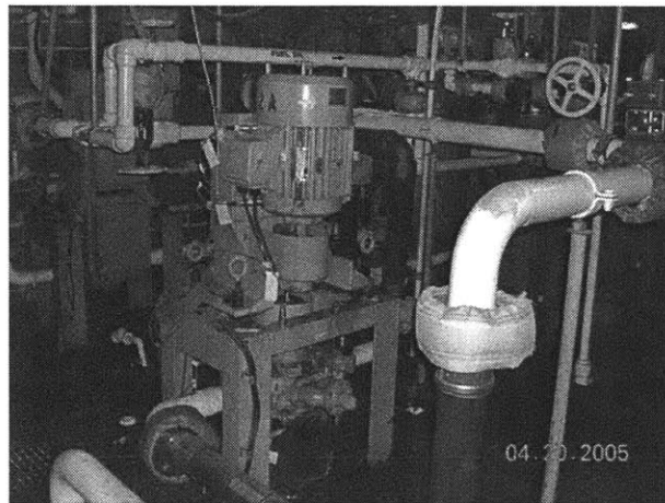
Figure 3-5: LBES Fuel Service Pumps.
