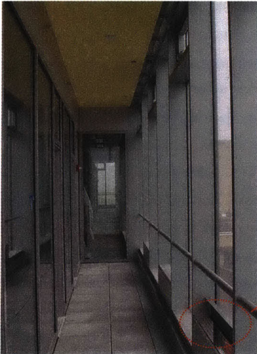
Figure 46: The vents could be better sealed with a rubber strip to prevent infiltration of cold air in winter.
