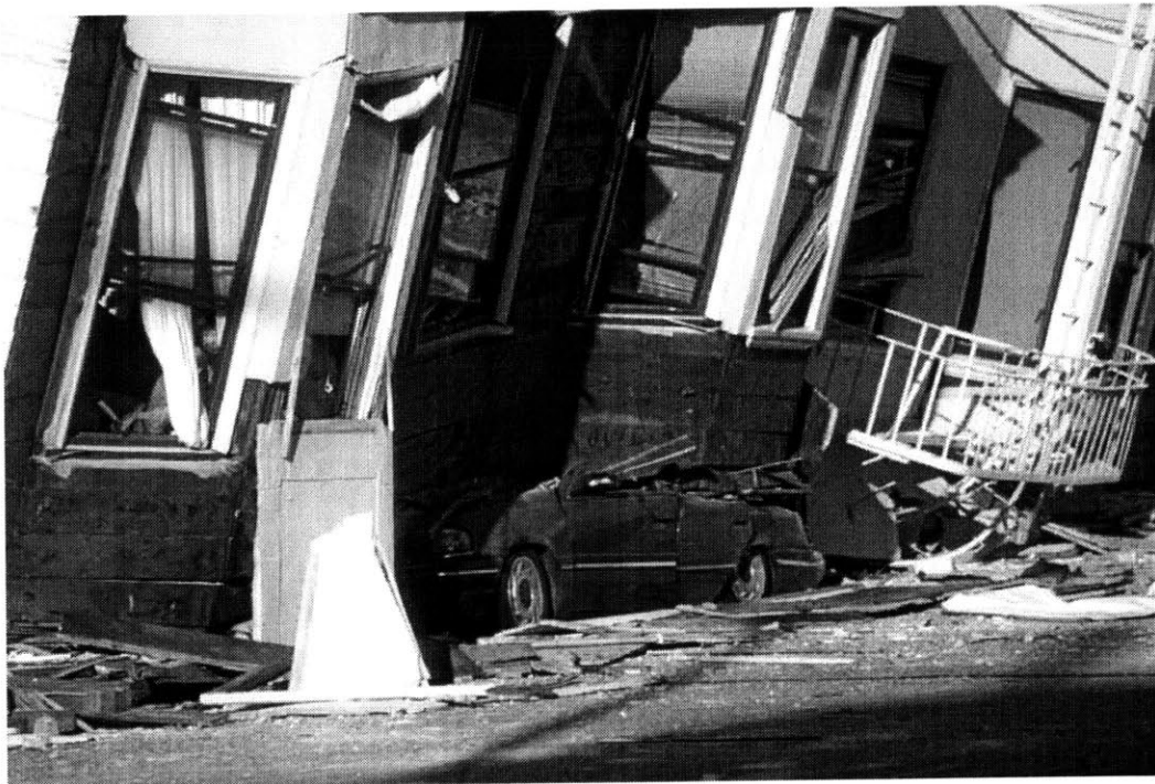
Figure 1.1 Damage Due to Northridge Earthquake 14
