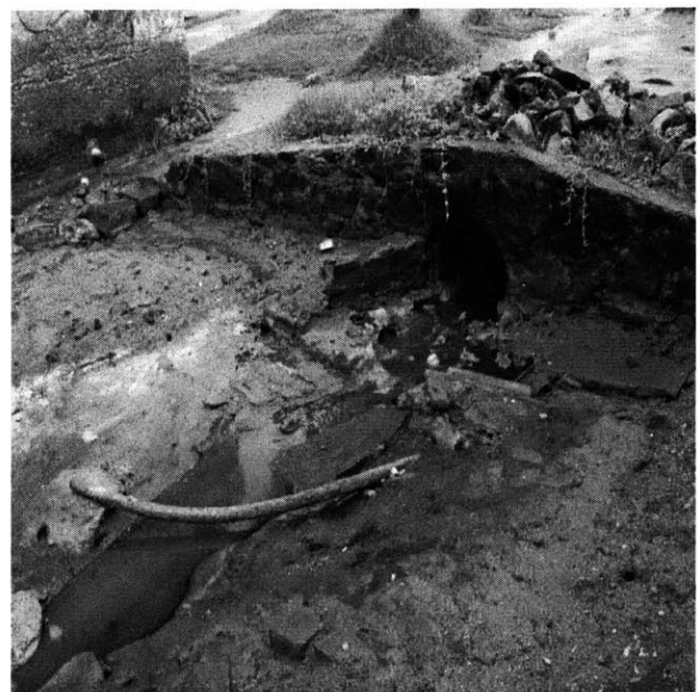
Figure 1.6: Sewage Discharge into street (1)
