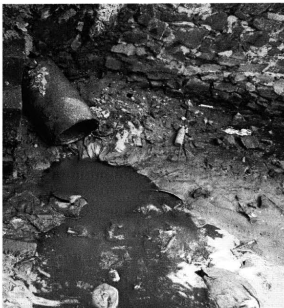
Figures 1.5: Sewage Discharge into stream
