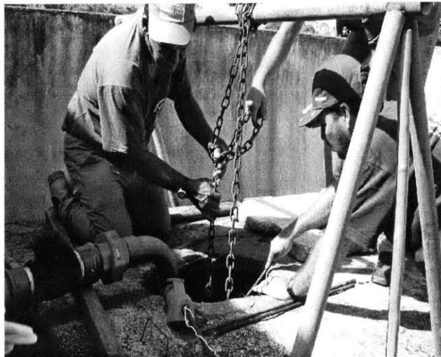
Figure 1.11: Collecting sewage from a tank
