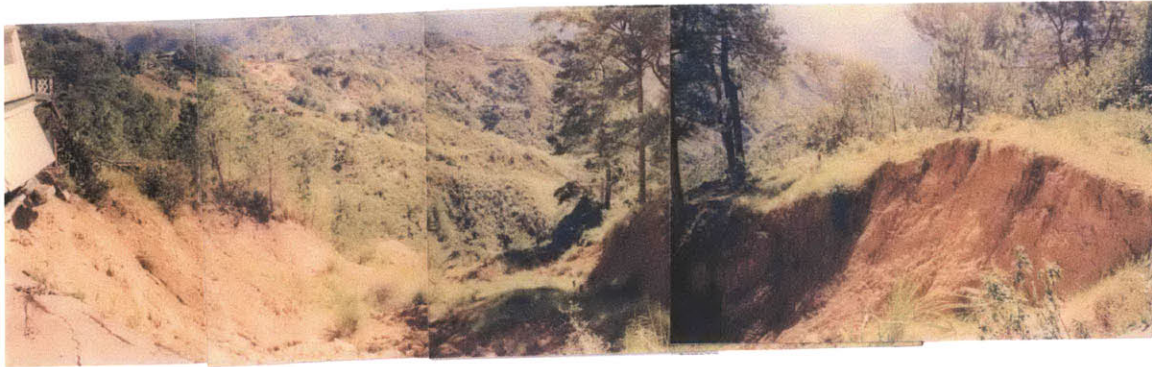
Figure 3.8 View of Slope Failure from its Crest (Geotecnica, 1987)
