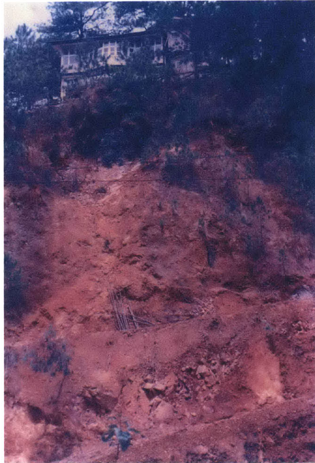
Figure 3.11 Front View of Landslide (Geotecnica, 1987)
