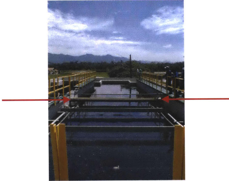
Figure 12: Scum Scraper Located at the Surface of the Clarifier Tank
