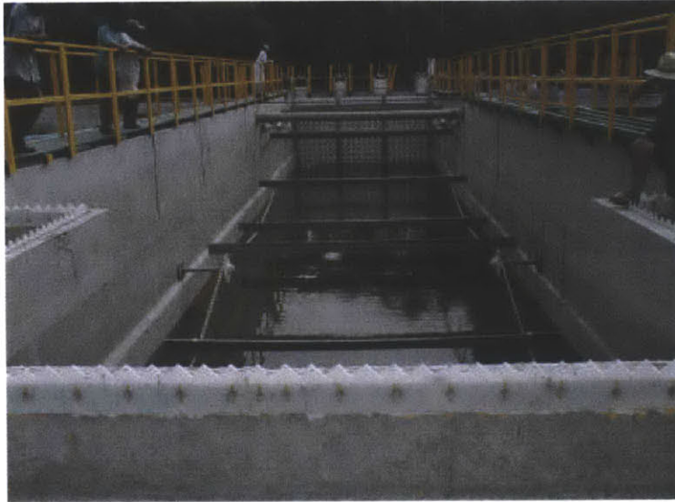
Figure 11: CEPT Tank and the Sludge Scrapers
