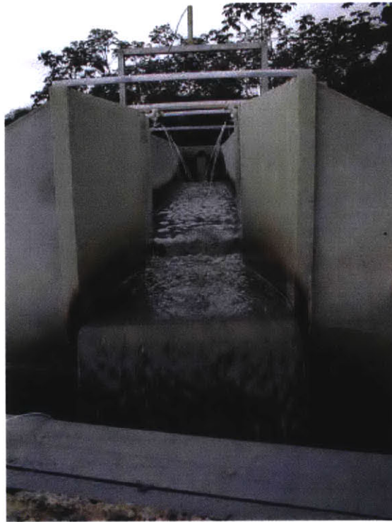
Figure 22: Sampling Point I-2, Influent Parshall Flume
