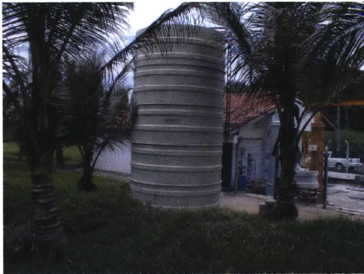
Figure 16: Chemical Storage Tank
