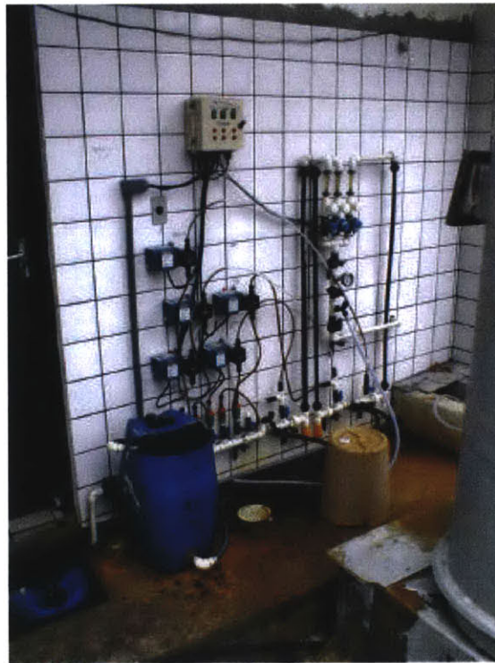
Figure 17: Metal Salt Dosing System
