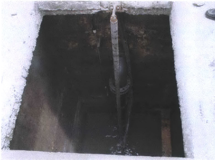
Figure 18: Metal Salt Injection into the Pump Well
