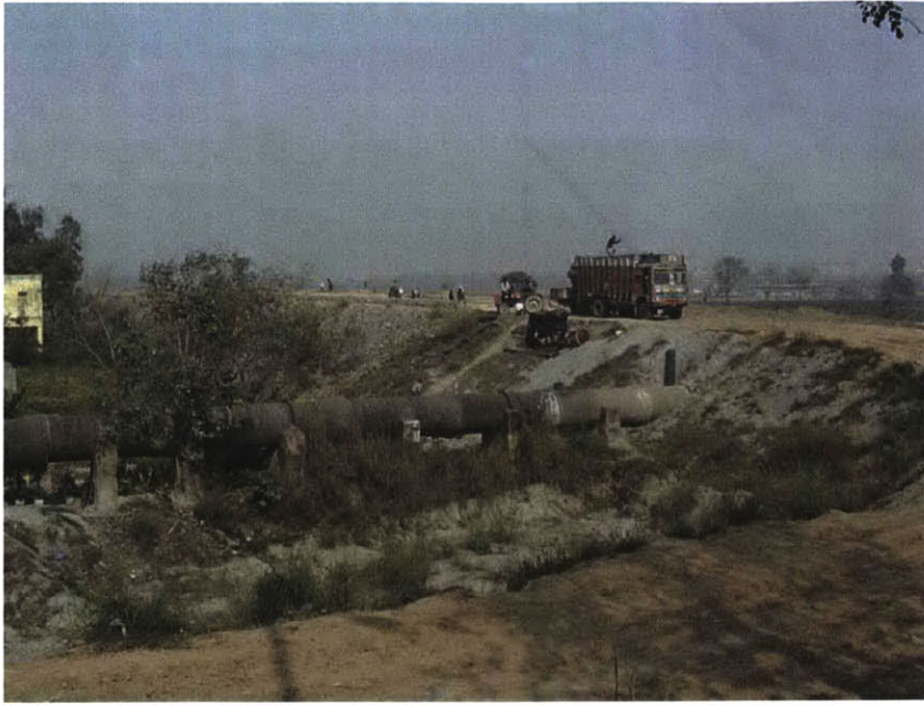
FIG. 1-4. Construction of Access Road to the Proposed CWG Village Site. The road is being built atop an existing flood embankment. Note the sand deposits from recent river floods, and the elevated
