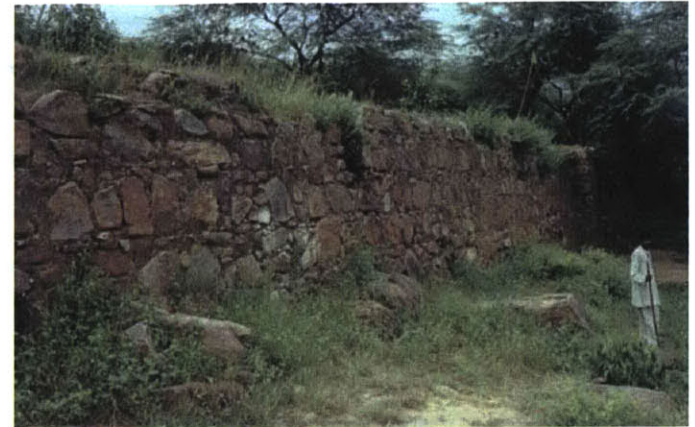
FIG. 2-12. The Talkatora Bundh , showing Rubble Masonry of the Dyke. The bundhs have survived largely as a result of the care ensured in their water-proof construction.
