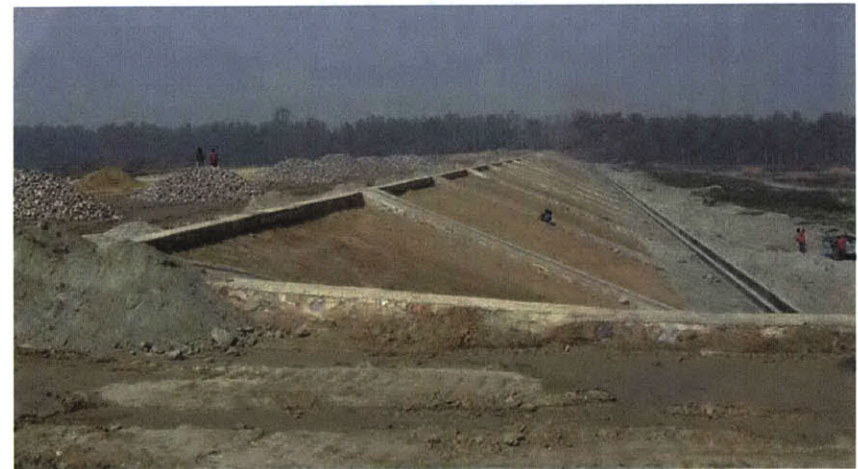
FIG. 1-7. The Worrisome Level Difference Between Road Level and Ground Level at the CWG Village Site
