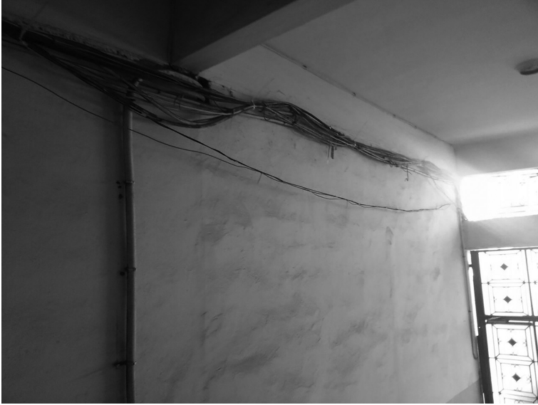
Figure 2.1 Diesel generator wires visible in the foyer of an apartment building in Beirut.
