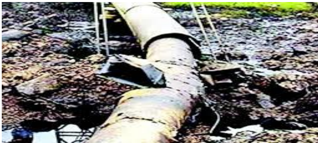
Figure 3.7: Vandalised crude oil facility
