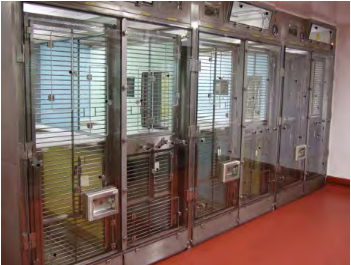
Figure 5 - A large animal directional flow containment system; pictured with NHP cages
