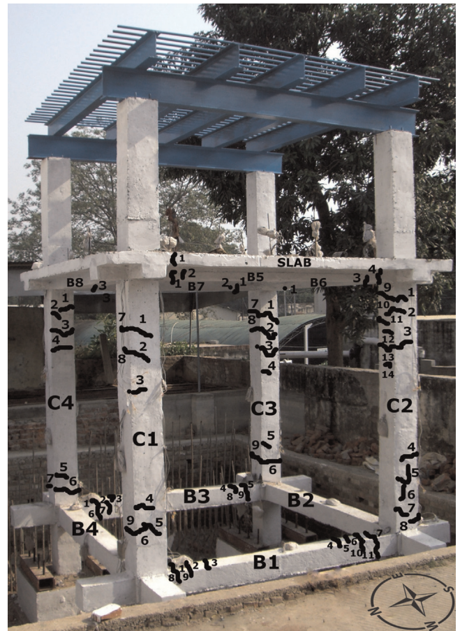
Fig. 8. Nomenclature for the identification of RC test frame members and schematic of cracks due to cyclic loading.
