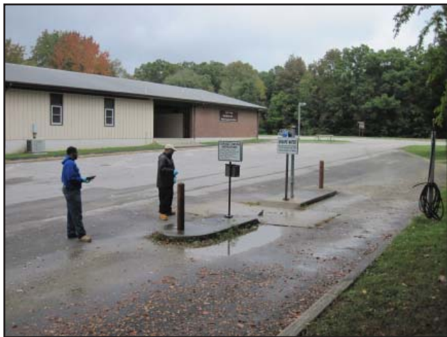
Figure 1: Storm-water drains from the Post Office parking lot and mixes with spilled waste residue, rich in QAC, at the RV disposal station. It carries the QAC into the storm filter, down the ravine, and into Annette's Dome (Cave level B). This drain area needs to be re-designed to prevent chemicals from getting into the cave.
