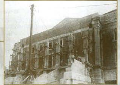
In fall 1910, construction on the Administration Building was proceeding slowly to the great consternation of President Cherry. The building was barely ready in time for Western's move to the Hill. (S. G. Rogers)
