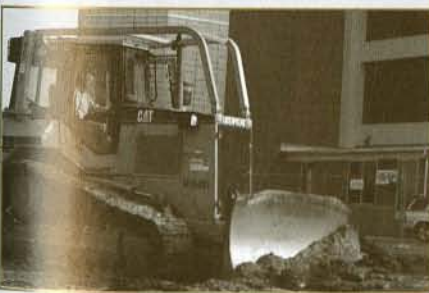
On Sept. 13, 2004, President Gary Ransdell took the helm of a bulldozer to break ground for a new 824-space parking structure between E.A. Diddle Arena and L.T. Smith Stadium. (Sheryl Hagan-Booth)
