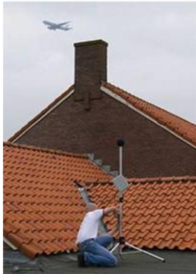
Figure 1. Installing a measurement point of the sensor network. Source: Alderstafel Schiphol (2012).
