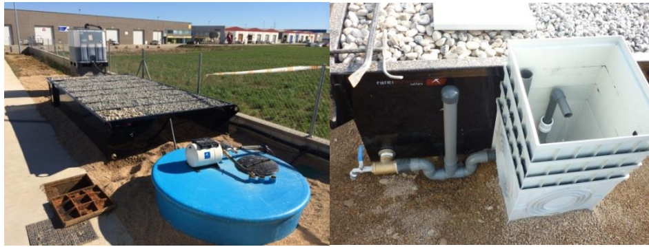
Figure 5.7. HFCW container and outlet device
