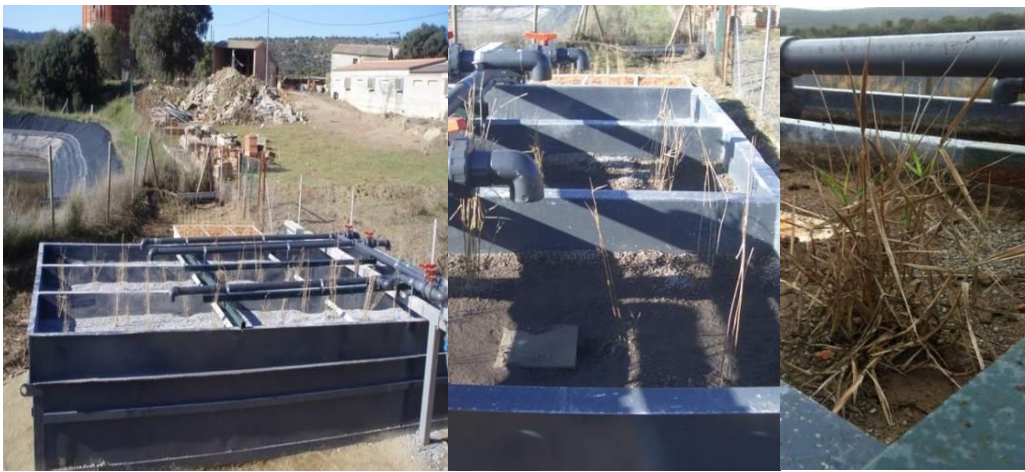
Figure 4.5. VFCW pilot: general view, distribution pipe and Phragmites australis
