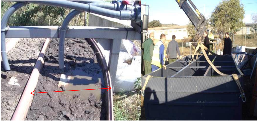
Figure 4.4. First VFCW tank with problems of lateral pressure and the new tank
