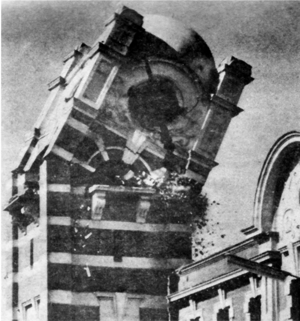
Figure 3. The clock tower coming down in 1969 (Taranaki Newspapers 1976:35) (Courtesy of Taranaki Daily News ).
