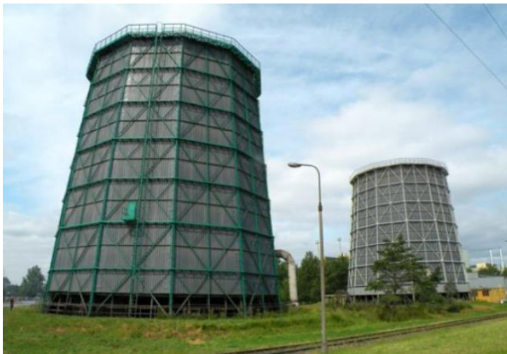
Figure 24: Steel NDDCTs are not constrained to the conventional hyperbolic shape, the towers shown are at the Celsa Ostrowiec Steelworks ("Cooling Towers: Overhaul of two natural draft cooling towers in celsa ostrowiec steelworks ", 2007) in Poland.
