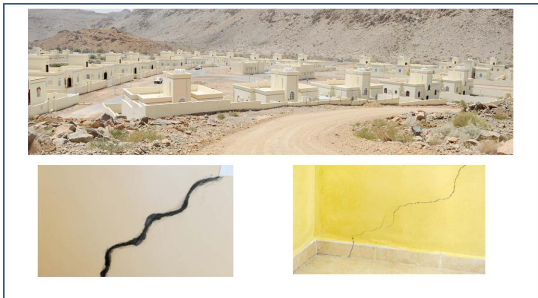
Figure 4.2: Cracks on social housing units’ walls
