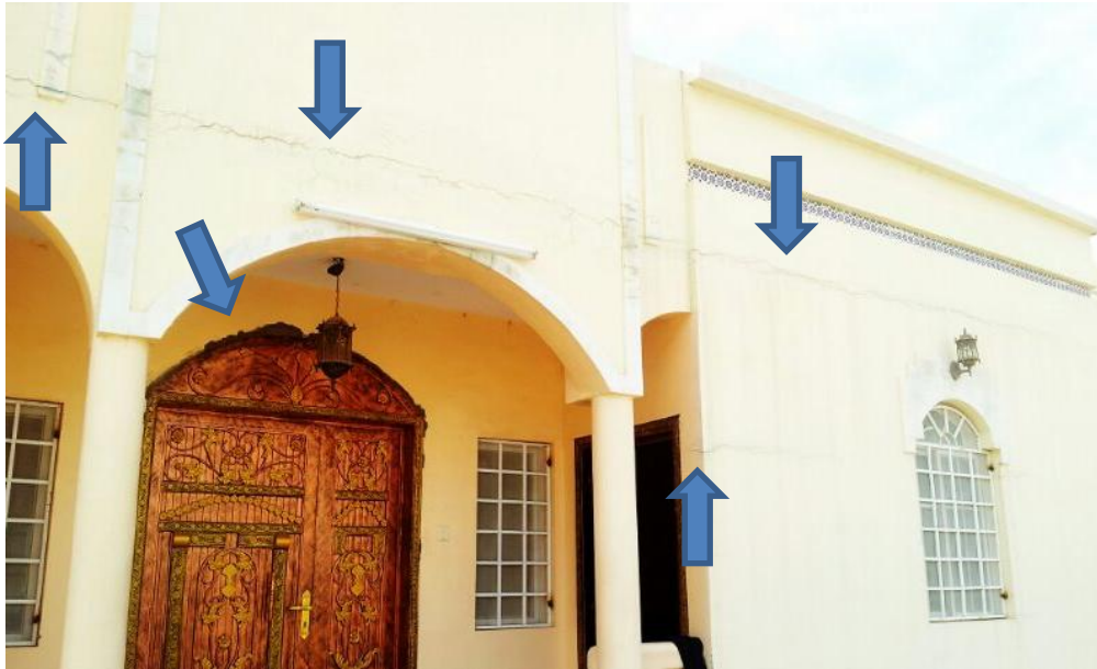
Figure 6.17: Cracks on social housing unit's walls and doors in Wilayat Nizwa
