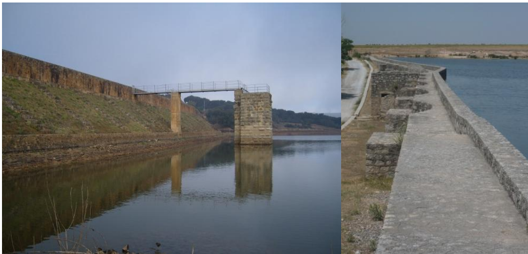
(A, Left) Cornalvo dam, Spain with the intake tower in 2007 (Courtesy of Franz Jacobsen)
