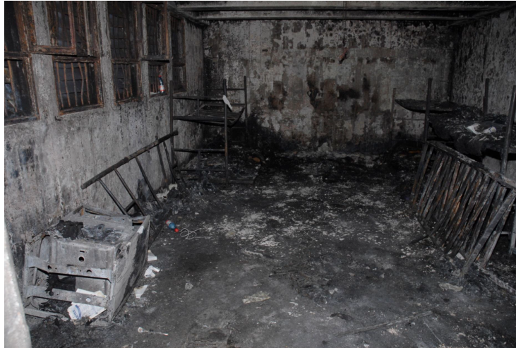
Figure 4: Post-fire internal view of the small room where the fire started.
