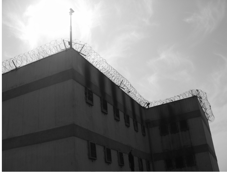
Figure 2: External view from north-east of Block 5 of San Miguel's prison. This photograph was taken a few days after the fire. The CCTV camera that captured the smoke coming out of the windows of the sanitary facilities on the day of the incident can be seen in the upper part of the image.
