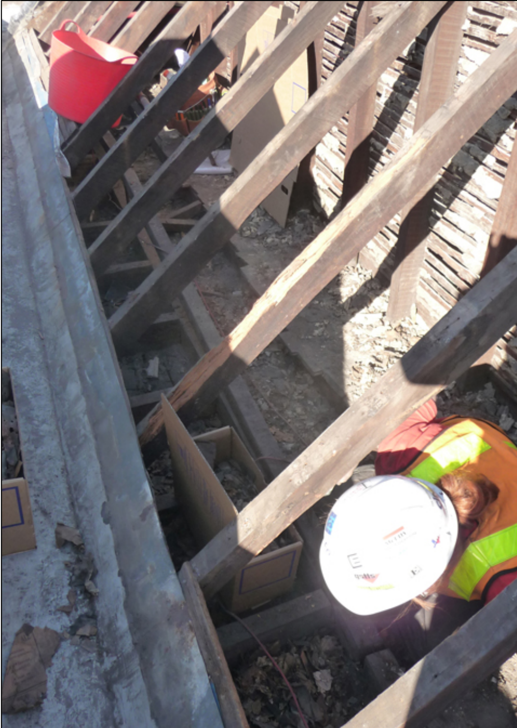
Figure 9. View of northern crawl space of 109 George Street where the rats nest was located (Photo courtesy of Sydney Harbour Foreshore Authority 2009).
