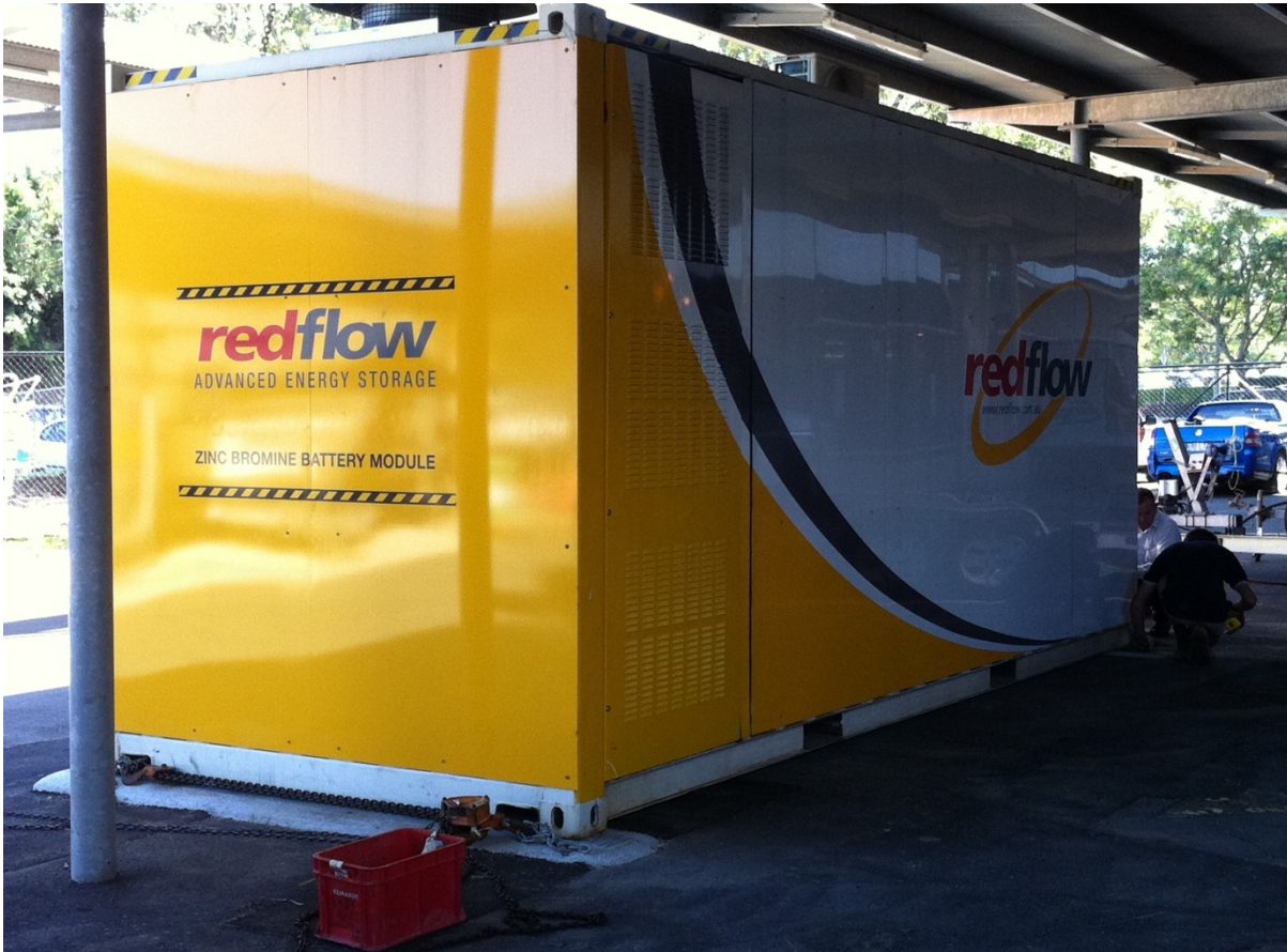
Figure 41: Red Flow Battery (April - 2011)
