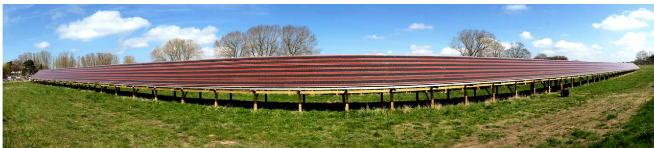
Fig 5.1 – Picture of the solar park at DTU. Reprinted with permission from 1.
