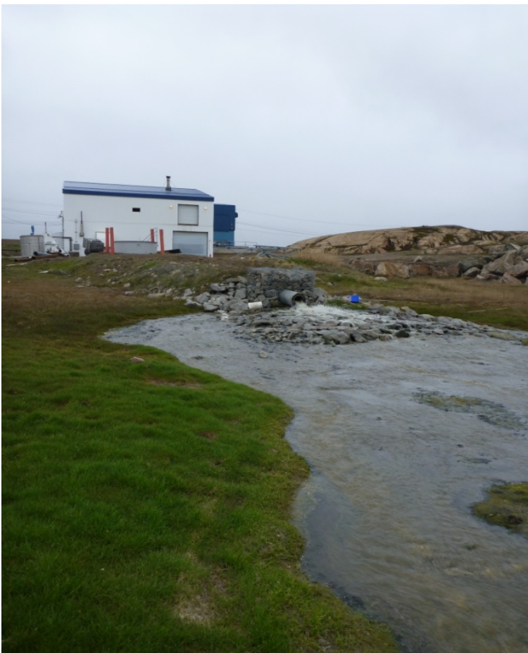
Figure 1. Mechanical wastewater treatment system in Iqaluit, Nunavut
