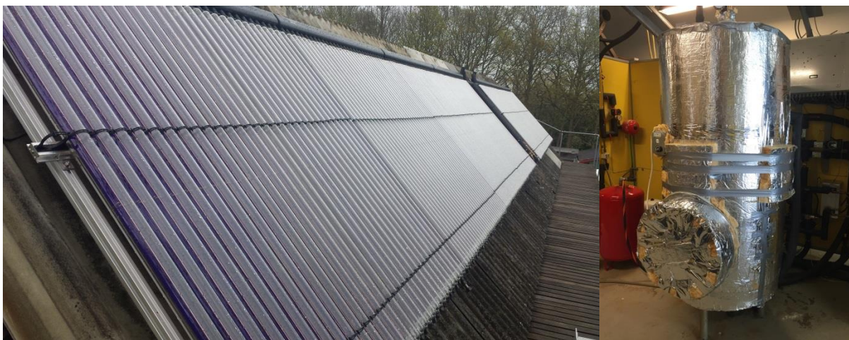
Figure 28. (a) Evacuated solar collectors for demonstration system. (b) 735 liters water buffer storage for demonstration system.
