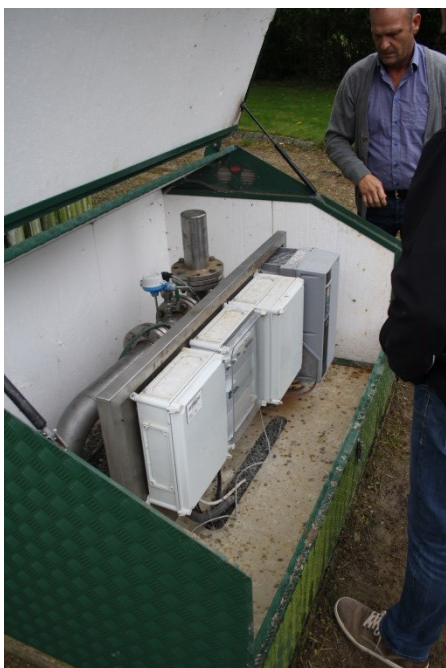
Figur B5-1 Pumpestation.
