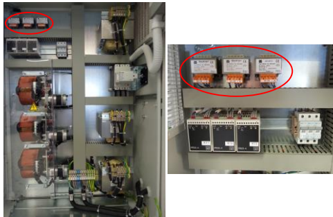
Fig. 11. Three single-phase Measurement Transformers
