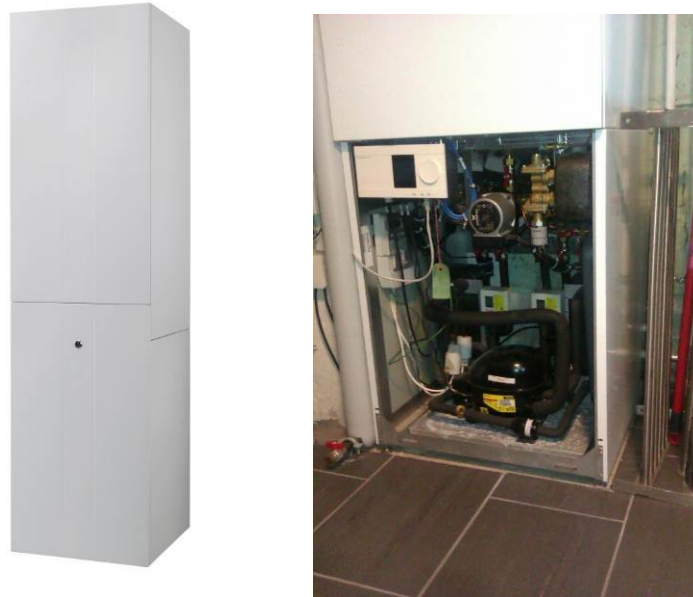
Figure 5: Left: Cabinet, tank placed in the top part and heat pump, controls, heat exchanger, electronic controller and pipes in the lower part. Right: Lower part of heat pump unit.
