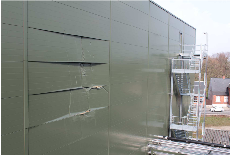
Figure 4 The tank rose almost vertically in the air and the base of the tank rose higher than the 19 m tall green building. Whilst descending, the tank impacted and deformed the building's exterior wall panels (Photo courtesy: Frank H. Hedlund)
