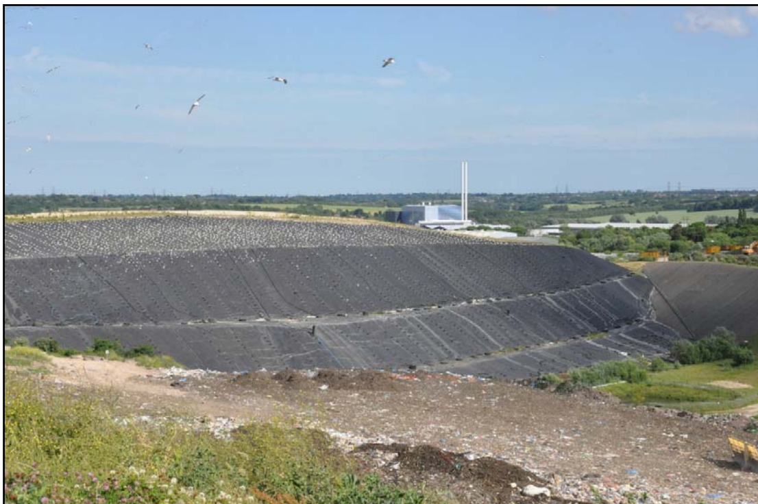
Figure 3. Photograph facing south east from the fully restored area of the landfill. The operational area where waste is being deposited can be seen to the right and foreground, and the area partially restored with a liner is shown in the centre.
