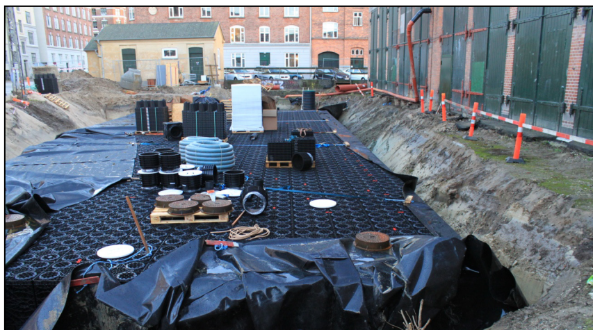
Figure 1. Construction stage of an infiltration trench in Nørrebro (Copenhagen). Photo from December 2014.
