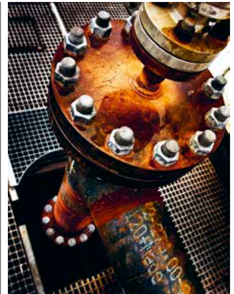
Geothermal heat is delivered directly from the underground to the district heating grid.
