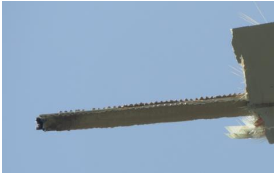
Figure 3-22. Tip detachment. The spar (load carrying structure) broke at several meters from the blade tip.
