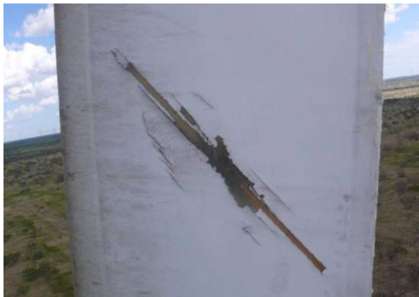
Figure 3-19. Delamination on the shell at about 2m from the blade tip due to lightning direct strike. It is observed how the fiberglass plies of the shell are detached around the strike point.
