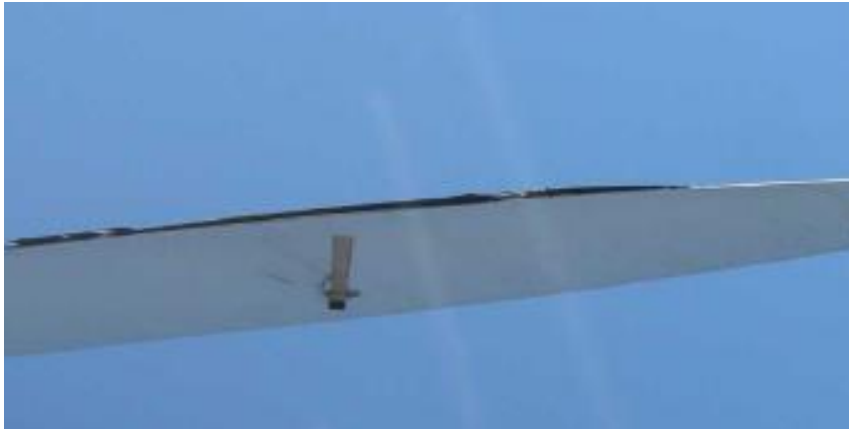
Figure 3-20. Delamination on the shell over the cap and debonding of the trailing edge likely caused by the expansion of the air caused by the lightning current.
