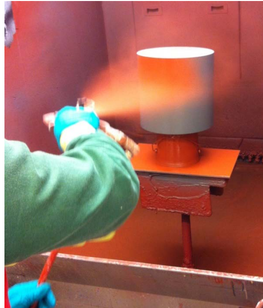
Figure 49A. Top-coat application on cylinder with airless spray. Primer is seen as the grey coating.
