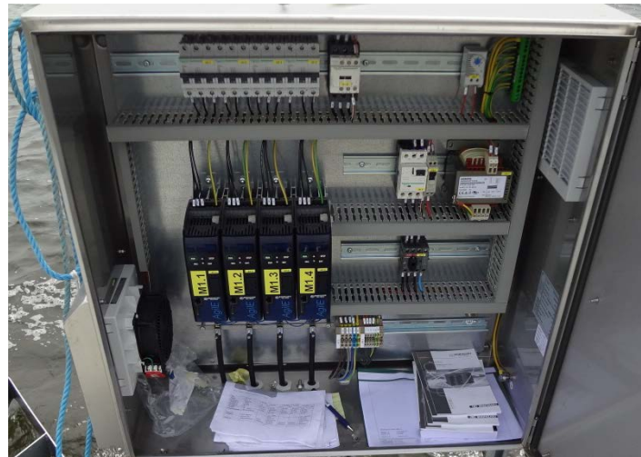
Figure 30A. Frequency converters M.1.1, M1.2, M1.3, M1.4 and electrical cabinet.
