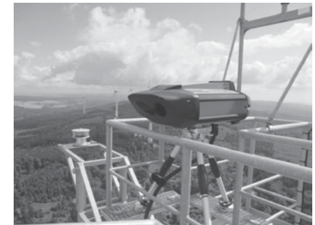
Fig. 1: Wind Iris multi-range pulsed LiDAR installed on turbine roof
