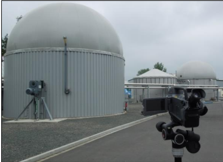
Figure 1: Infrared camera during use on the exploratory biogas plant of the DBFZ
