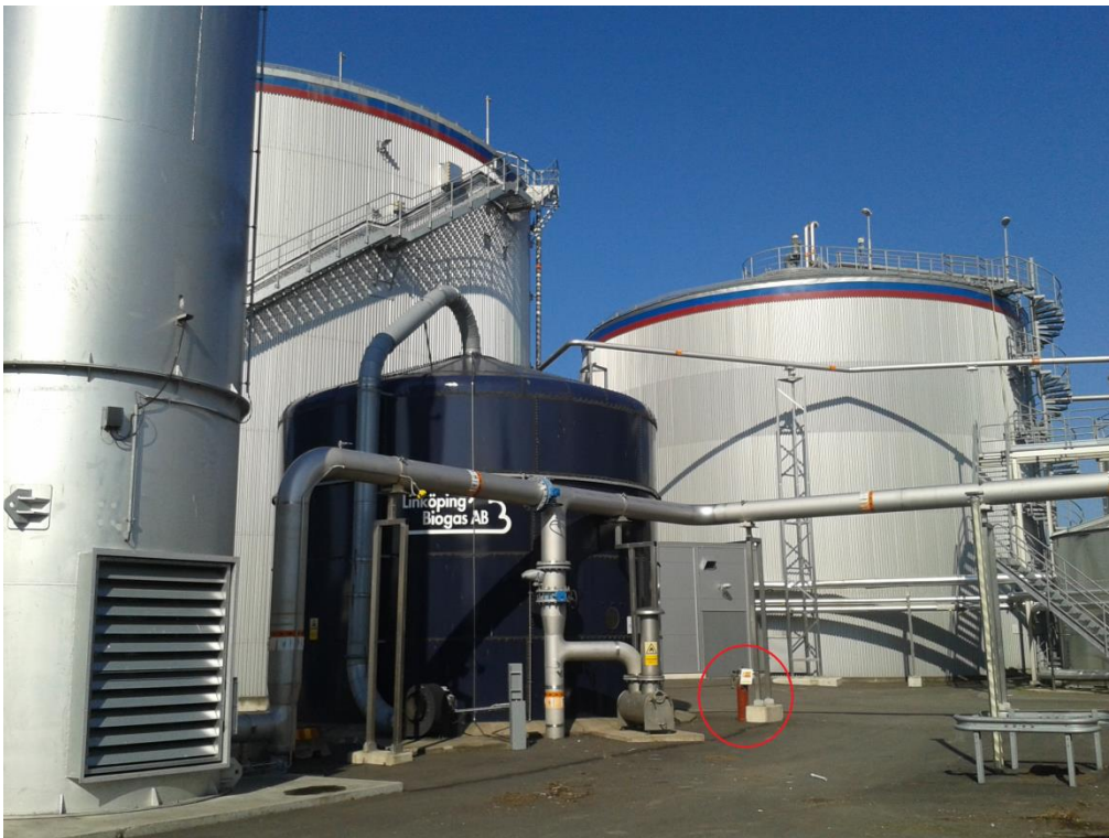
Figure 3. Acetylene cylinder placement close to digester tanks marked with red circle
