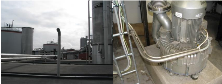
Figure 11 a). Overview of detected leakages, arrows indicate precise location of the leakages (taken from DGC report).
