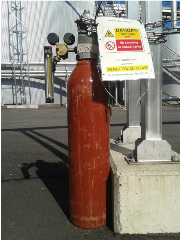
Figure 2. Acetylene cylinder secured at the digesters area
