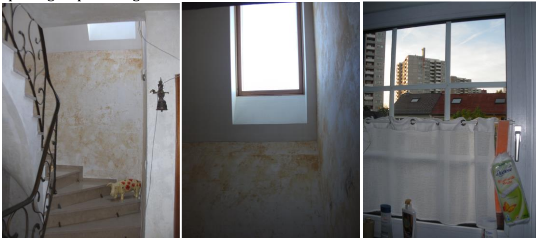
Photo: Hiltrud’s problematic window – and right: Barbara’s bathroom window which is never opened
