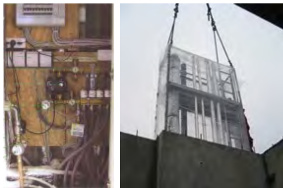
Figure 7: Installation shafts before and after the application of modularity as a tool for managing complexity.
