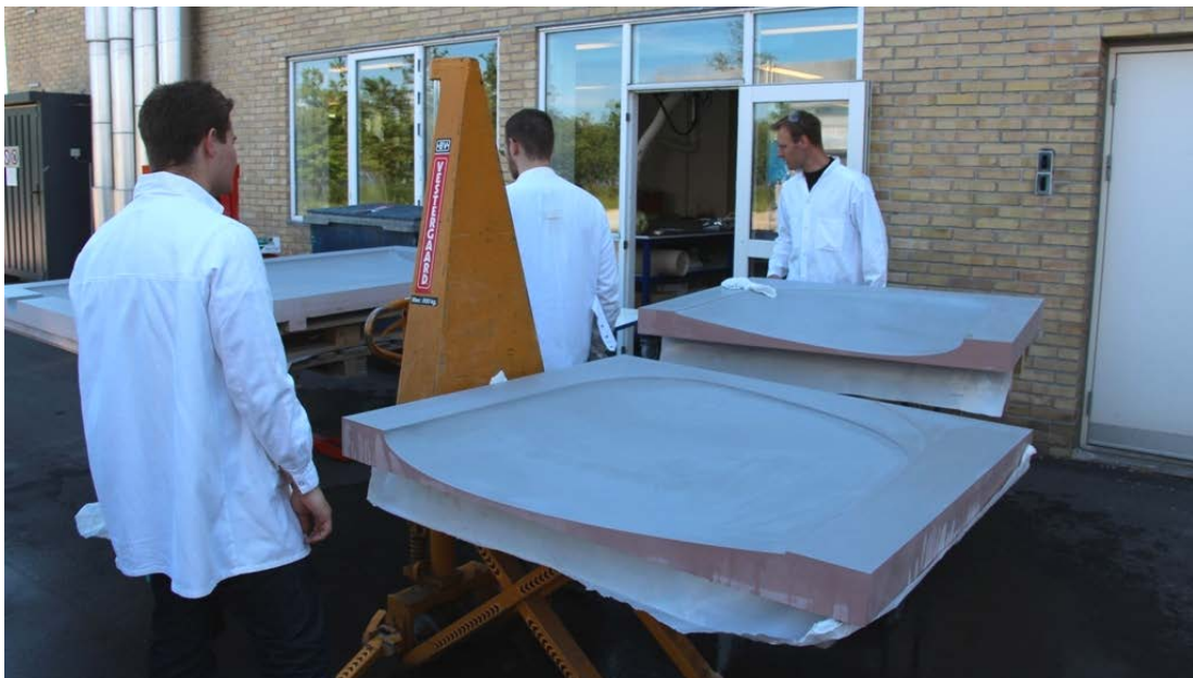
Figure 18 - Delivered molds were cleaned and treated with a release agent; Zyx Composite Shield delivered from Granudan (Stenløse, Denmark) and later on REXCO's wax PARTALL #2 delivered from R&G Faserverbundwerkstoffe GmbH (Waldenbuch, Germany).
