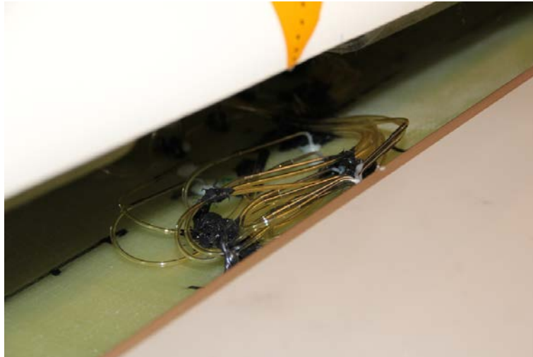
Figure 36 - Check of space and test of pressure tubes - all work before assembly.
