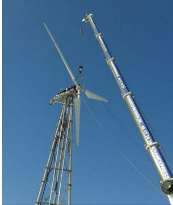
Figure 1 - The 100kW Tellus turbine at the Risø campus test field.
