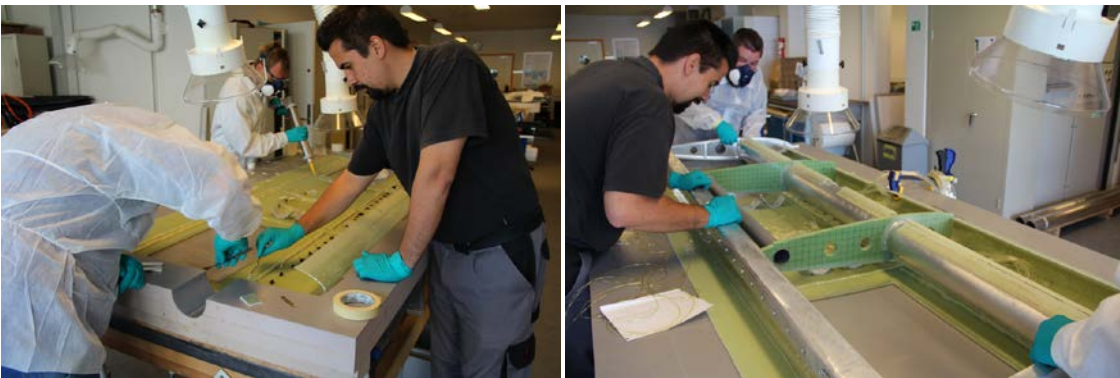
Figure 31 – Left: The adhesive was manually spread out before placement of the aluminium structure. Right: Careful placement of aluminium structure on top of composite shell.
