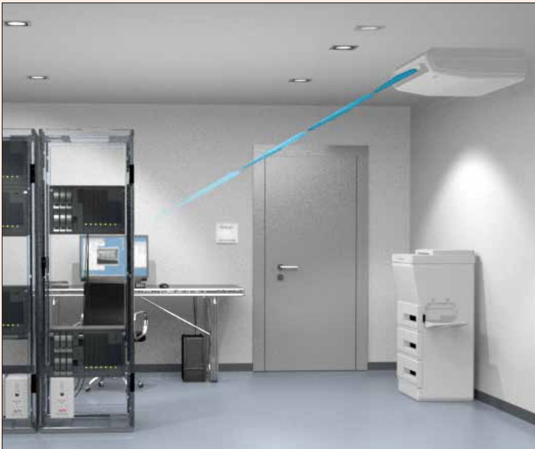
Precision and comfort air conditioners differ significantly in air flow rate and speed as well as in the control concepts.
